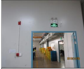
Photo of fire safety equipment 2. Emergency Light. Safety Exit Sign. Fire alarm. JPG
